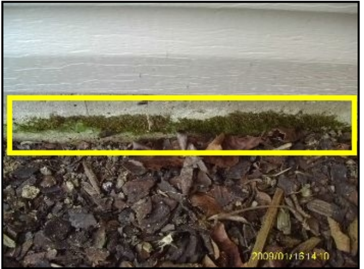
moss on foundation
