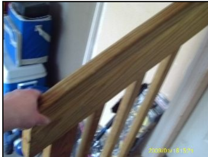
Loose railing on stairs in Garage
