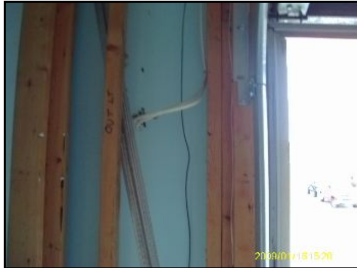
Exposed wiring with unfinished walls
