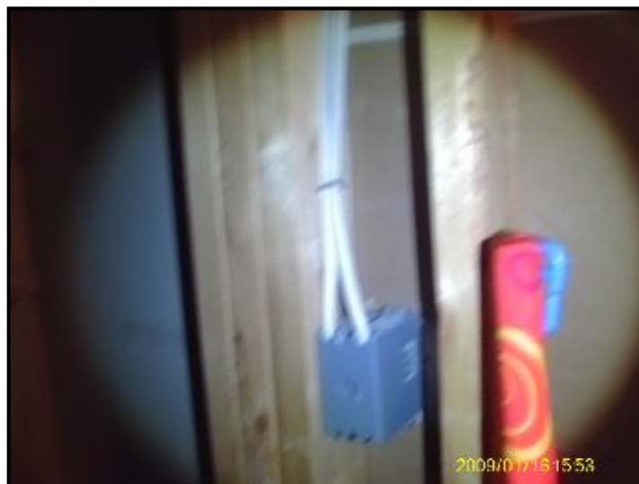
exposed wiring at a height accessible for children
