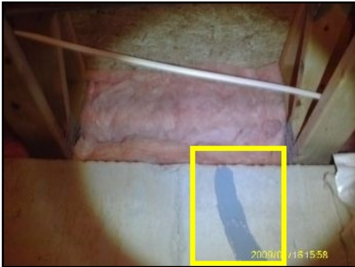
Previous repairs made
