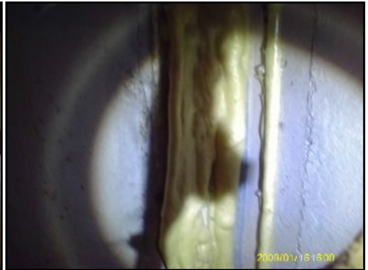
Covered with Spray insulation to cover crack
