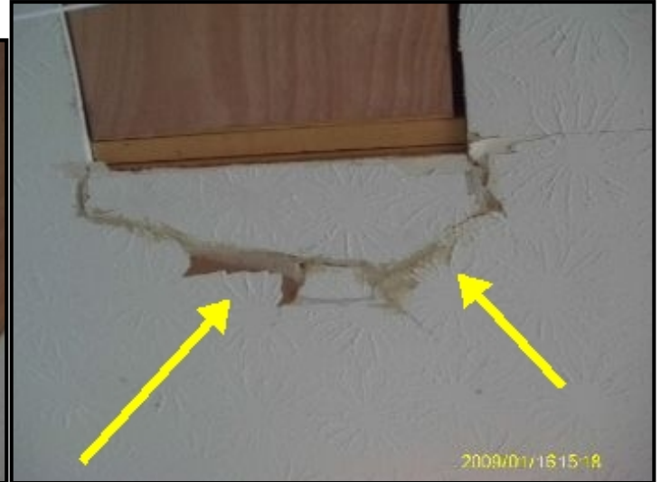
Ceiling cracks - LARGE
