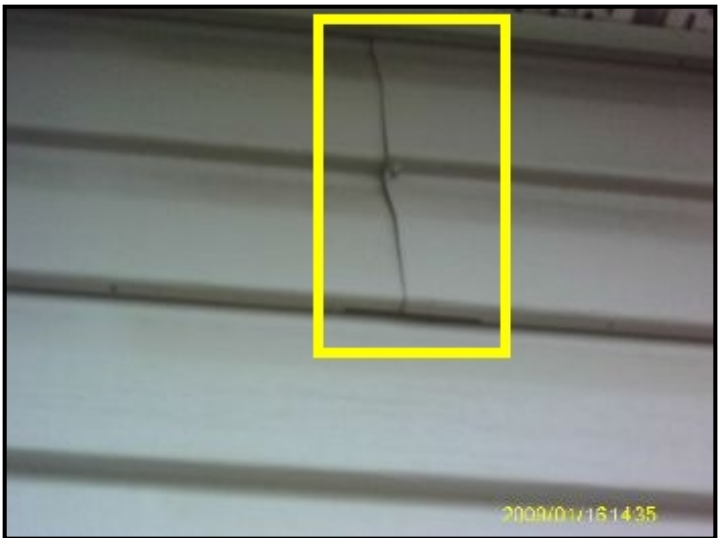
Needs nailed down - too open to the elements
