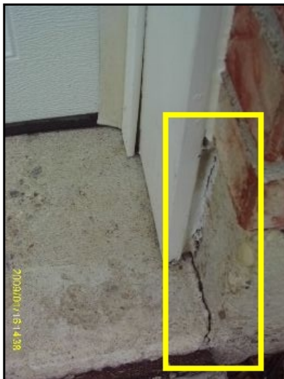
Area needs sealed
