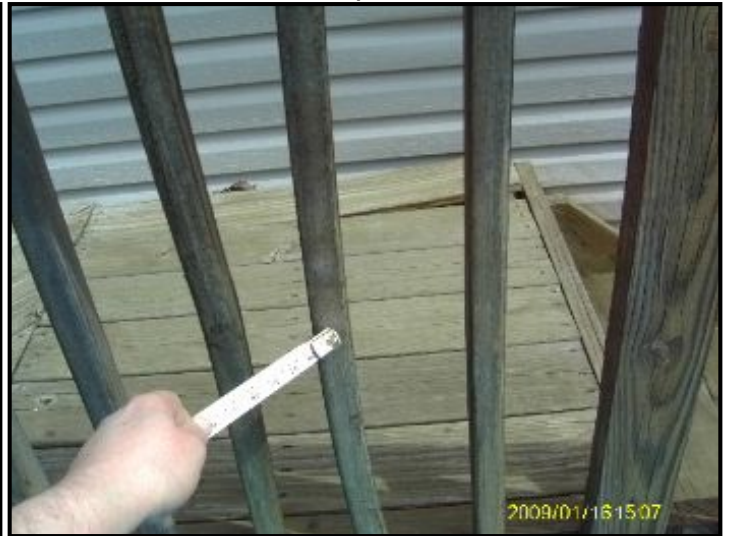
Balusters are bowed
